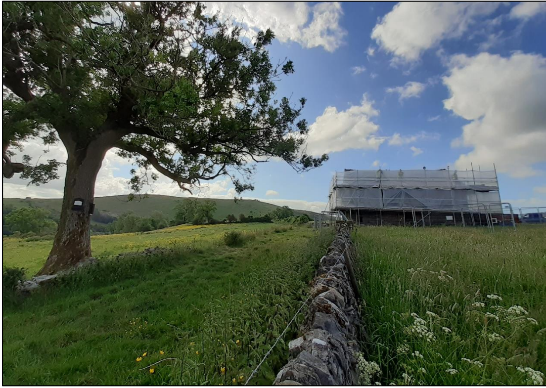
Fig. 13 mid works: the barn is covered in scaffolding and a bat box has been placed on a nearby tree
